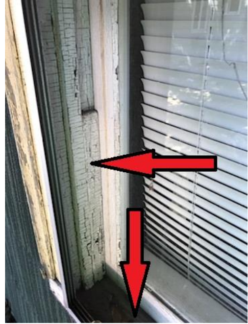
White painted wooden window jamb and gray well. This deteriorated paint, combined with the operable window, represents impact and friction hazards.
