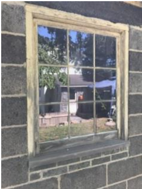
Yellow painted wooden window components on the garage. The paint used on these original windows are lead-based.
