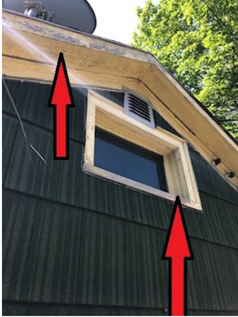
Yellow painted exterior wooden window components and trim. All of the yellow components are lead-based. The continued operation of the window makes this a friction hazard.
