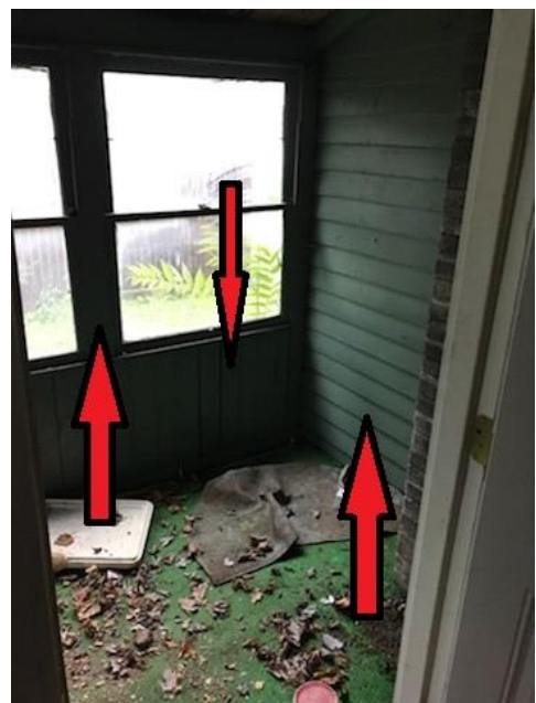
Green painted wooden porch wall and window components. The damage sustained to the components is evidence of weather exposure.
